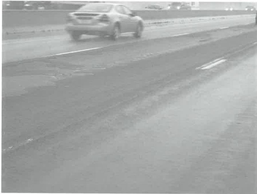
Figure 7. Delamination of Lane 2 Microsurfacing in 2004 after 4 Years in Service
