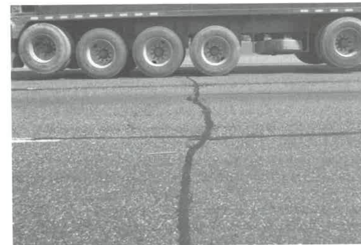
Figure 7. Sealed Transverse Crack in Stone Mastic Asphalt (SMA) Surface
