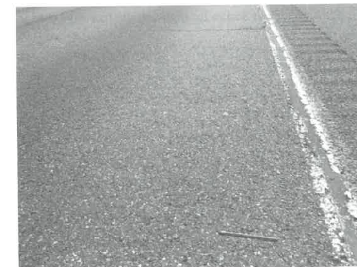
Figure 9. Raveling in Stone Mastic Asphalt (SMA) Surface
