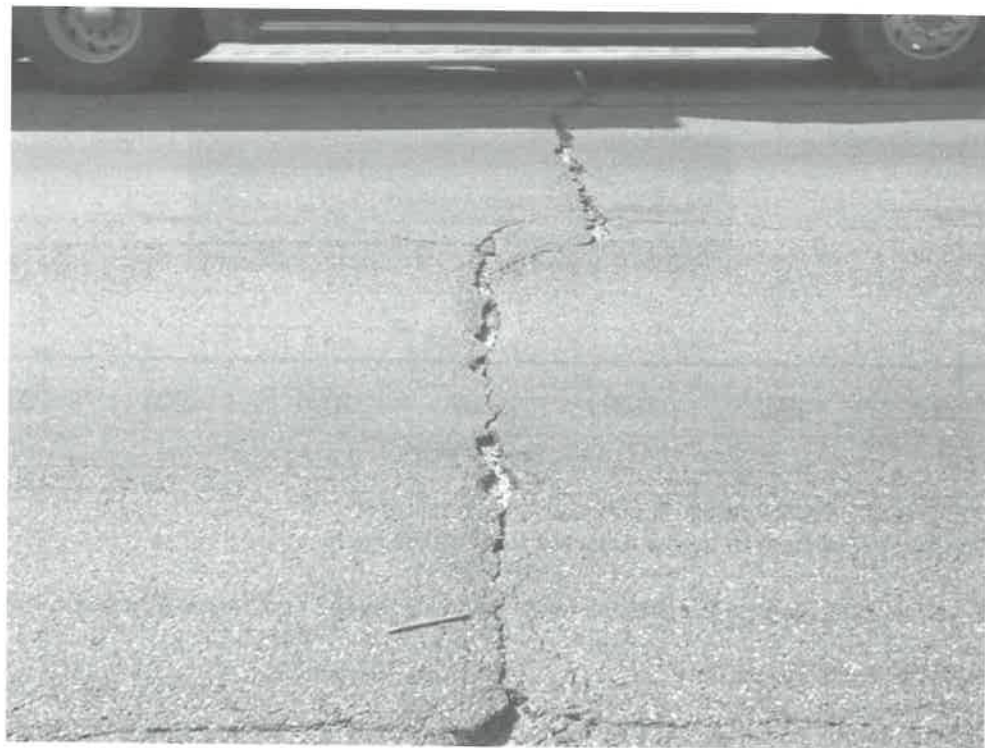
Figure 6. Typical Raveling of Transverse Cracks in Dense Friction Course (DFC) Pavement
