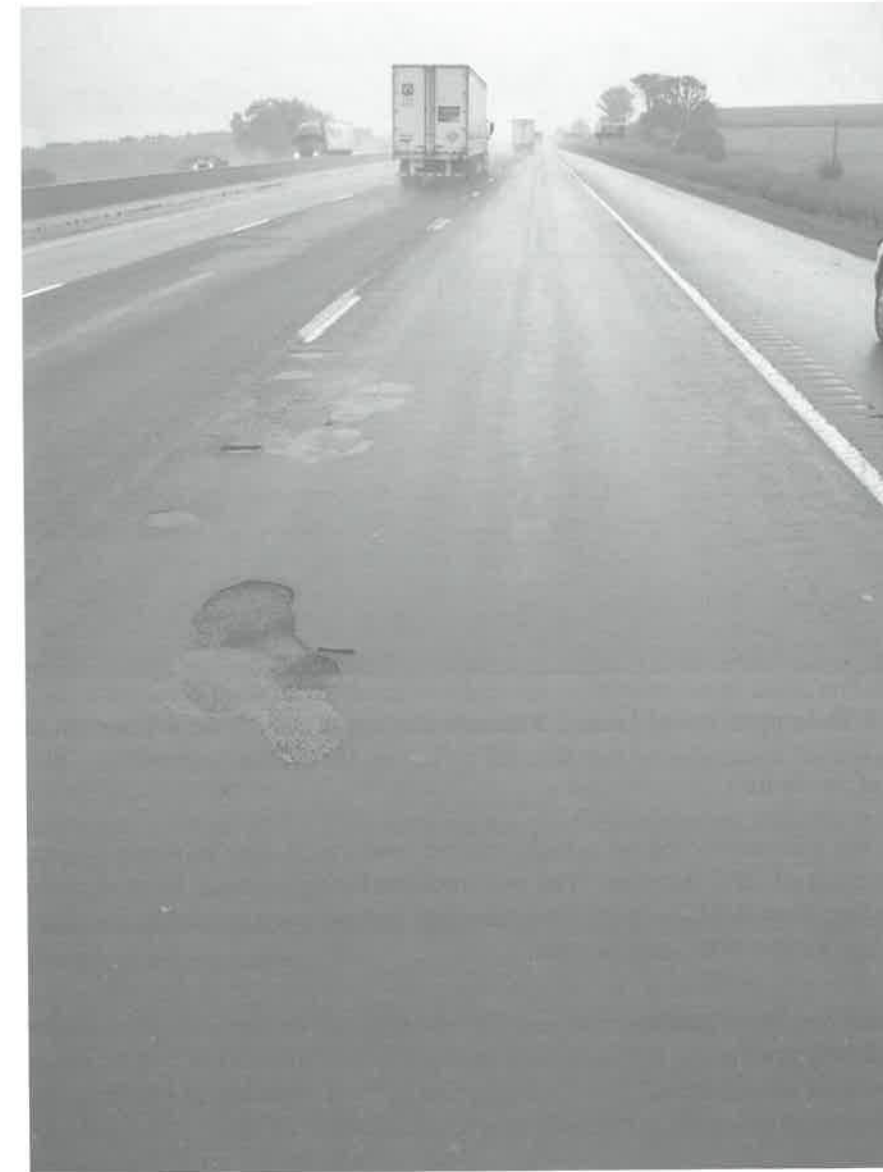
Figure 6. Severe Ravelling and Potholes in Lane 3 Micorsurfacing
