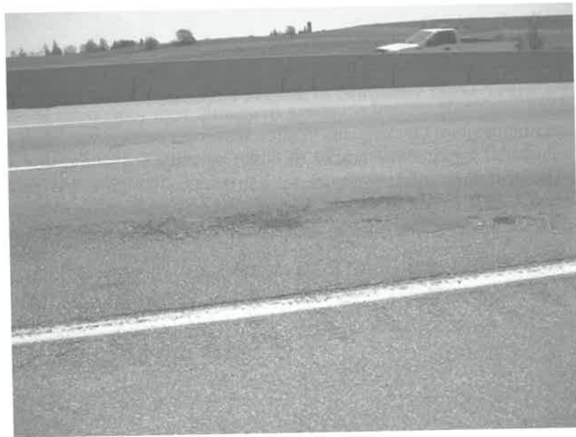
Figure 5. Potholes Appearing in RHM DFC Section
