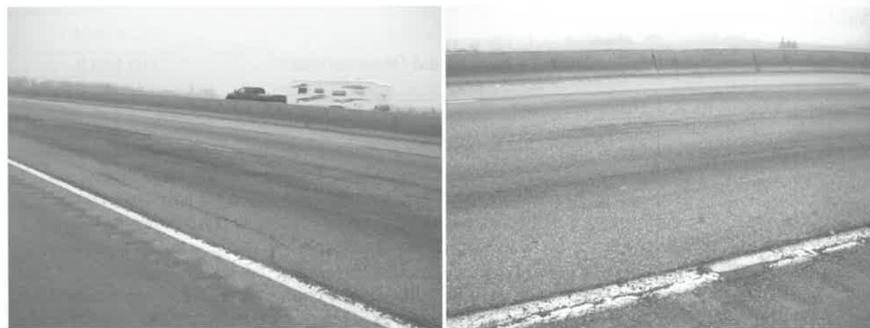
Figure 2. Distresses in Taisei HIR Section in 2007 after Eight Years in Service
