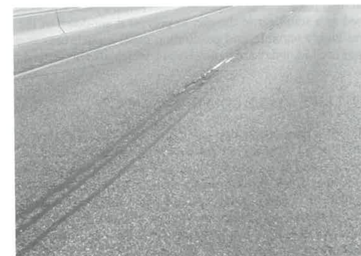
Figure 8. Sealed Longitudinal Joint, Exhibiting Multiple Cracks, Raveling, and Potholing in Stone Mastic Asphalt (SMA) Surface
