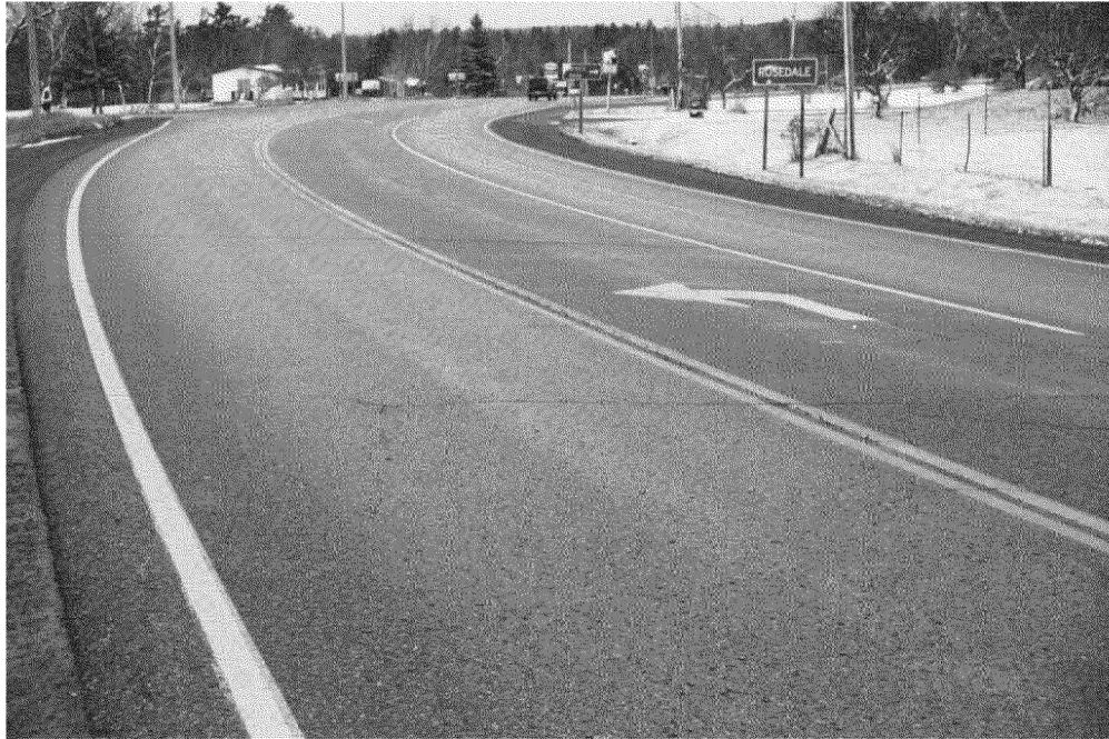
Figure 2 - Site 23 Slight Coarse Aggregate Loss
